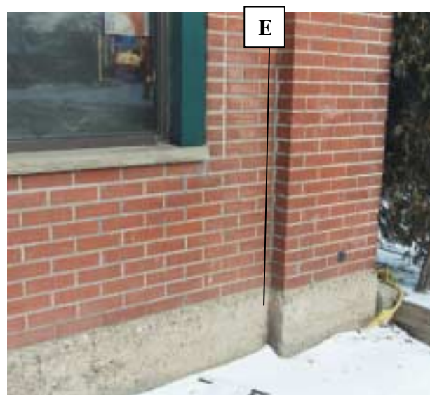
Figure 7 Pier adjacent to former garage opening E – Line between new & old masonry
