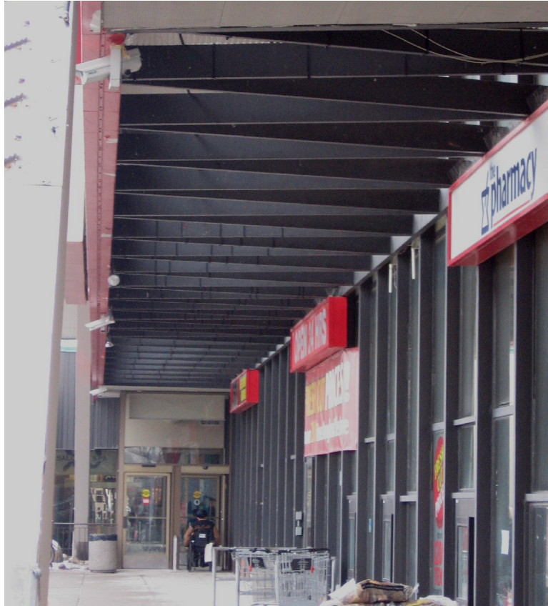
14. Photograph, Parkway Plaza, January 2008: showing the extended entrance canopy and, on the right, the lower part of the glazed north facade (Heritage Preservation Services)
