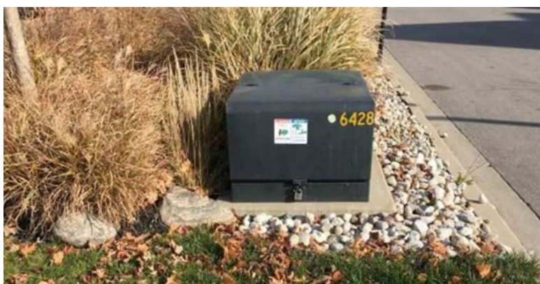
Padmount Transformer or Switchgear
